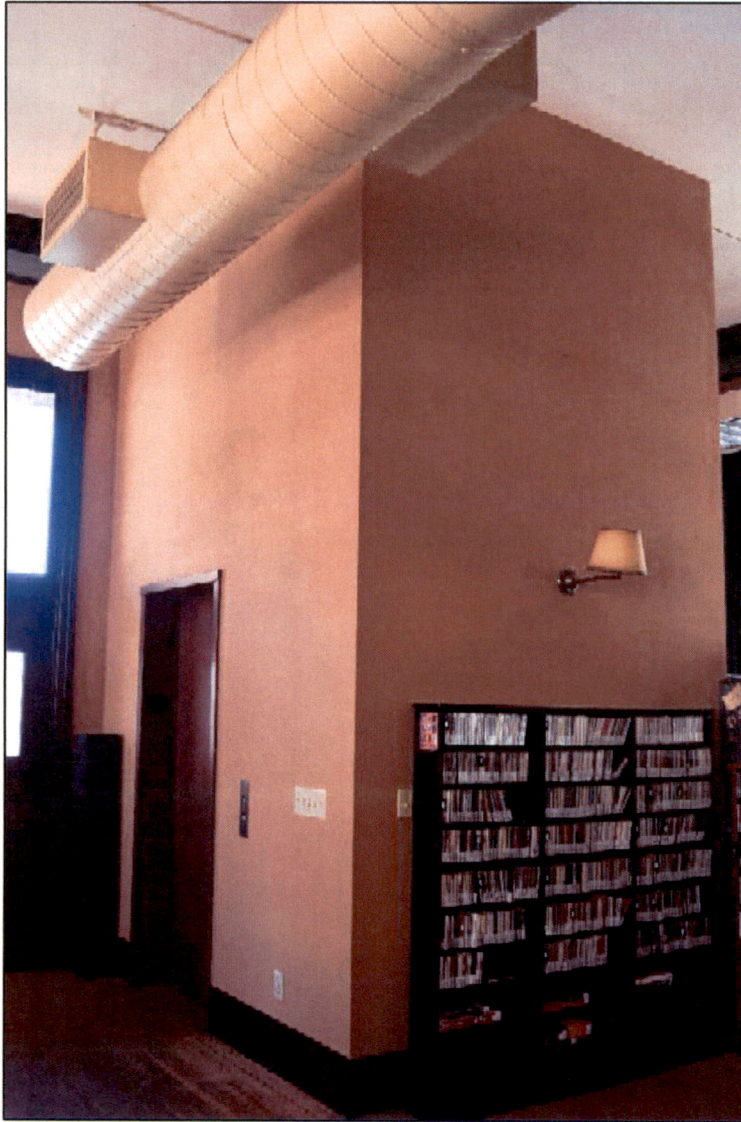
Figure 37. Modern elevator shaft and air duct, looking southeast. March 2021.
