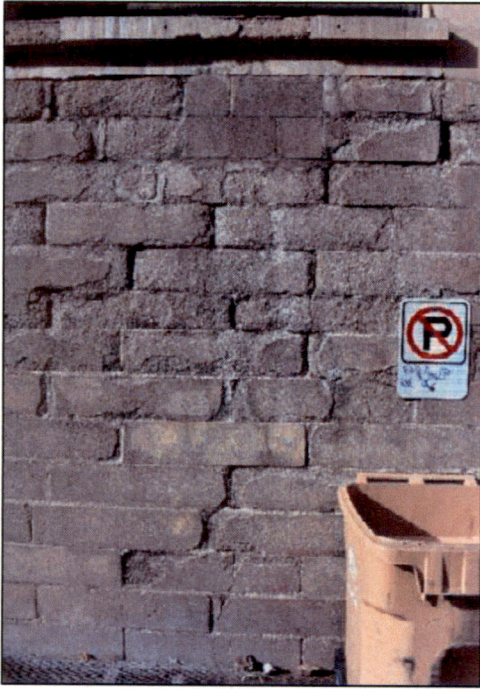
Figure 4. Damaged/undamaged gray smooth-faced blocks at ground story of south elevation. March 2021.
