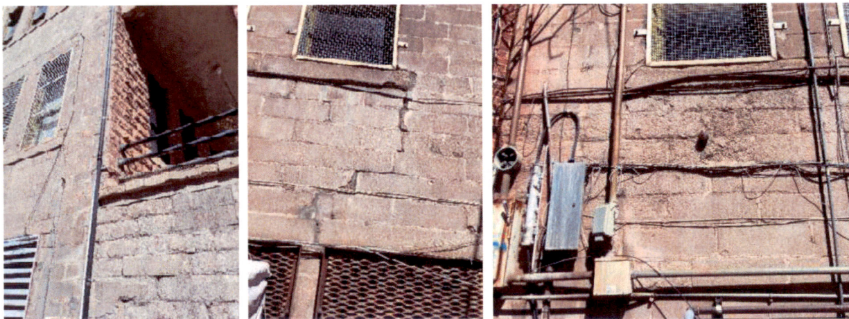
Unprotected and utilitarian south wall in need of more substantial repairs.
