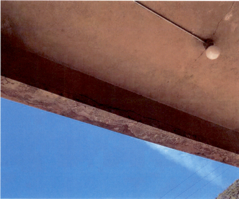
Photo 9 shows cracking in concrete beam s concrete porch deck. See elevation view for
